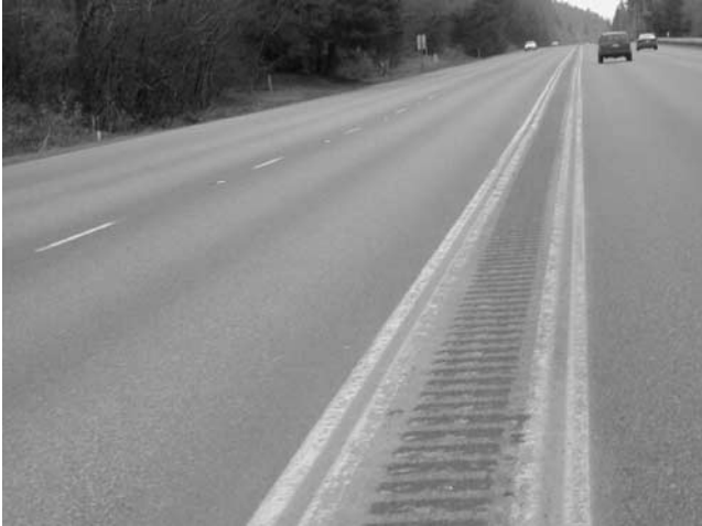
FIGURE 16 ODOT CLRS installed on Mt. Hood Highway (Source: Christopher.M.MONSERE @odot.state.or.us).
